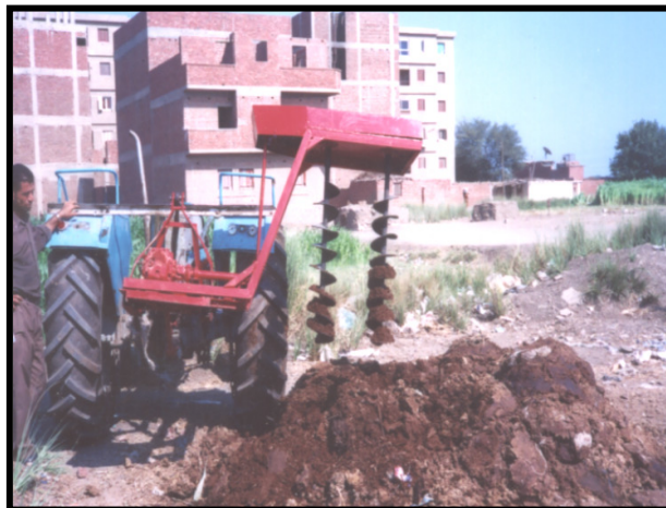
Fig. 7 : Upright turning machine during work on round pile .
