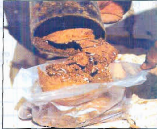
Fig. (3): P.V.C Trap after being buried into soil for 2 weeks
