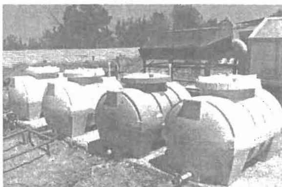
Fig. (1): Four water storage tanks used during the experimental work.
